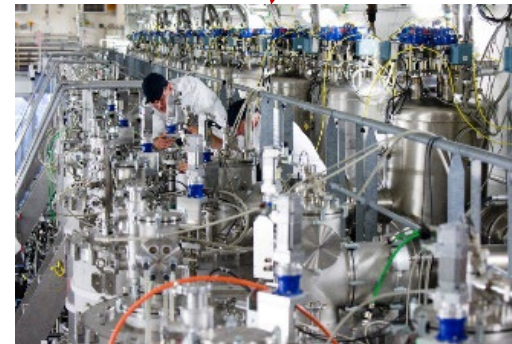
Cryogenic distribution system
