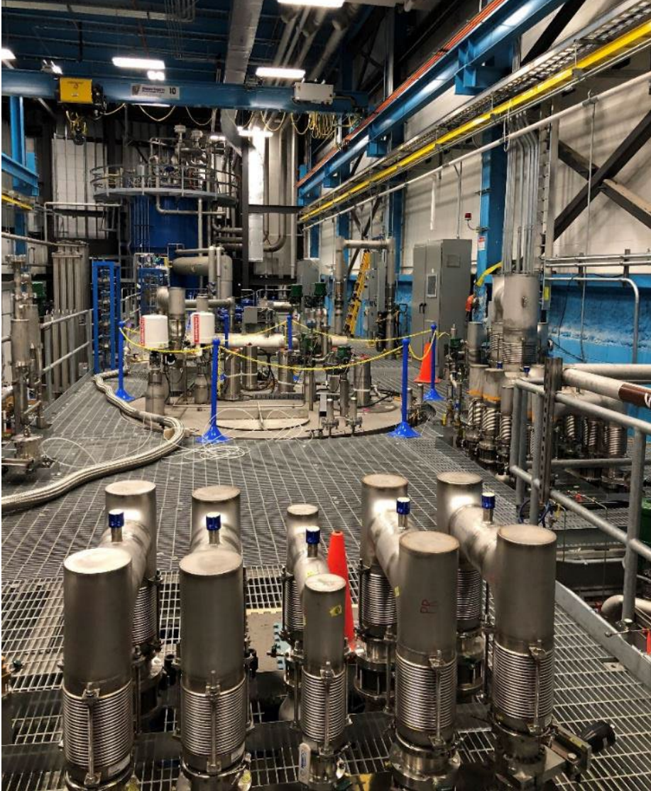
FRIB's state-of-the-art, high efficiency central helium refrigeration system
