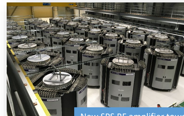
New SPS RF amplifier towers
