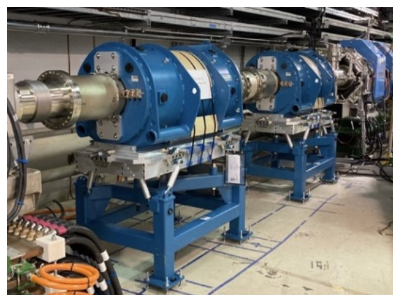
Figure 2: Solenoids installed in the SNS ring.
